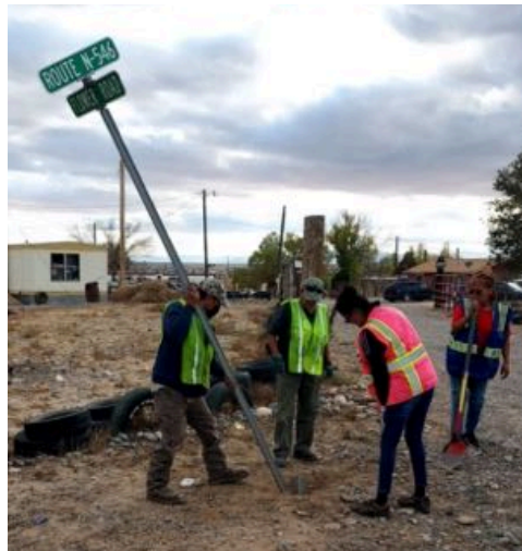
After the base post is installed, the assembled sign is mounted with the break-away assembly as part of the MUTCD (manual for universal traffic control devices) standards; BIA Roads and state highway department grant R-O-W (right-of-way) approval for the sign installations
