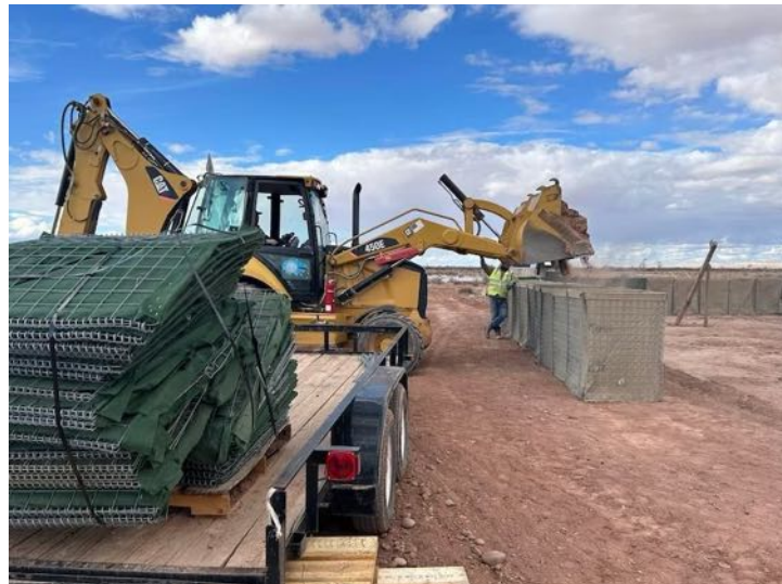
NAVAJO NATION DEPARTMENT OF TRANSPORTATION WORKS TO REPAIR WASHED OUT ROADS AND CULVERTS IN APRIL 2023
